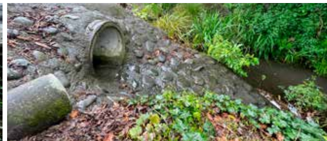
Stormwater infrastructure is conspicuous in the urban environment.
