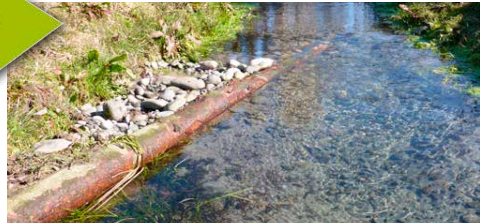
Log vanes are typically installed pointing upstream. Used in combination with bank reshaping to ensure that channel capacity is not reduced.
